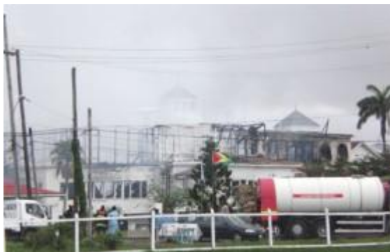
The hospital building after the flames subsided.
