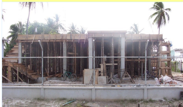
Picture of Tipperary Building construction taken March 28, 2011 Picture: Thanks to Fitzroy (Rollo) Younge .
